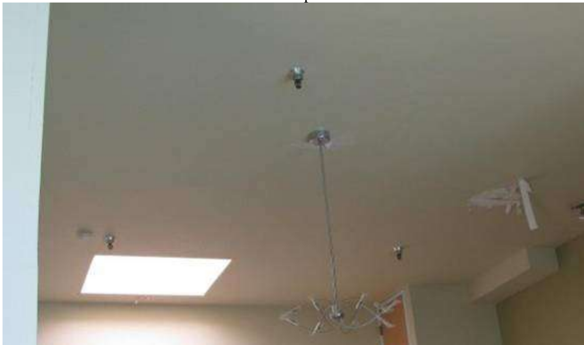
Figure 9 Visual view of room 304 ceiling
