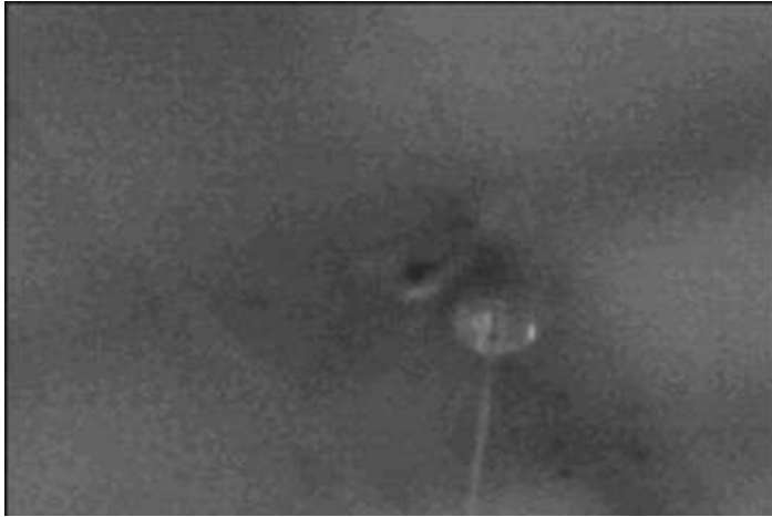
Figure 10a Thermal of light fixture joining ceiling
