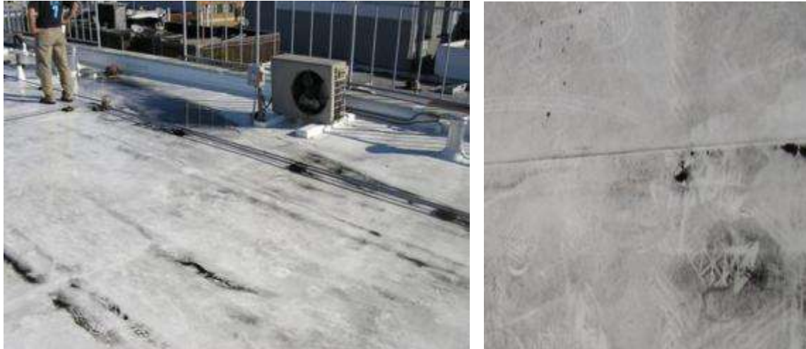
Figure 8 Water puddle on south roof and detail of roofing material seam
